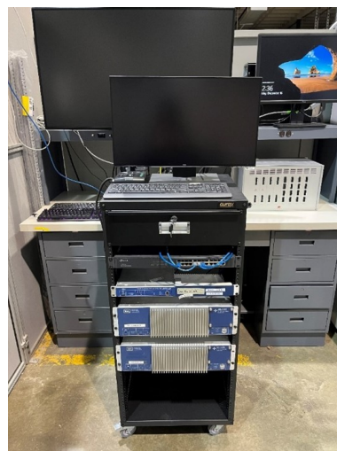
Figure 6. Strata Grid system in RPI Lab.
