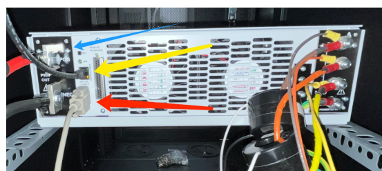
Figure 9. TDS-1000-15 DC power supply instrumentation and communications wiring. Blue Arrow: Output of DC power supply. Yellow Arrow: Ethernet Connection. Red Arrow: RS-232 Connection.
