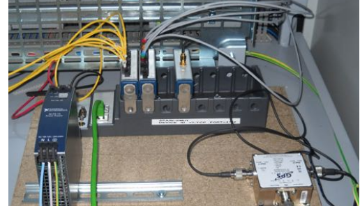
Figure 6. PMU installation layout at IREC 24V power supply (left), cRIO PMU (center) and GPS splitter (right).
